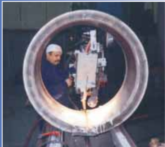
Submerged Arc welding of carbon, low alloy and stainless steel of all thicknesses.
